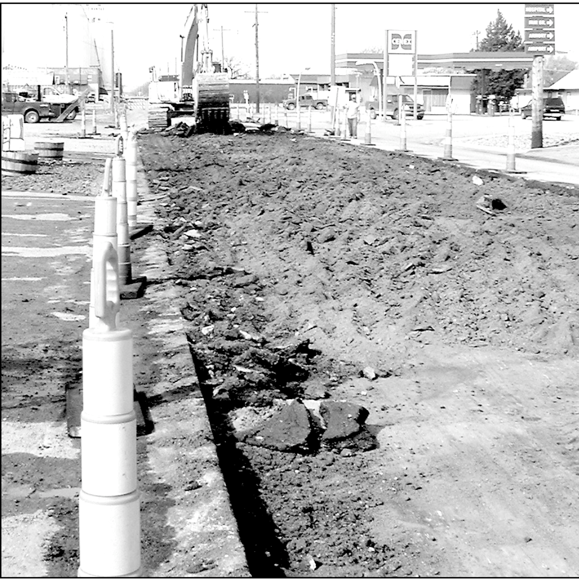
Sporer Land Development of Oakley began tearing out the asphalt from the south side of 17th Street from Cherry to Clark as the first phase of the street project began on Tuesday. The street is down to one-way traffic until the project is completed. Photo by Tom Betz/The Goodland Star-News
