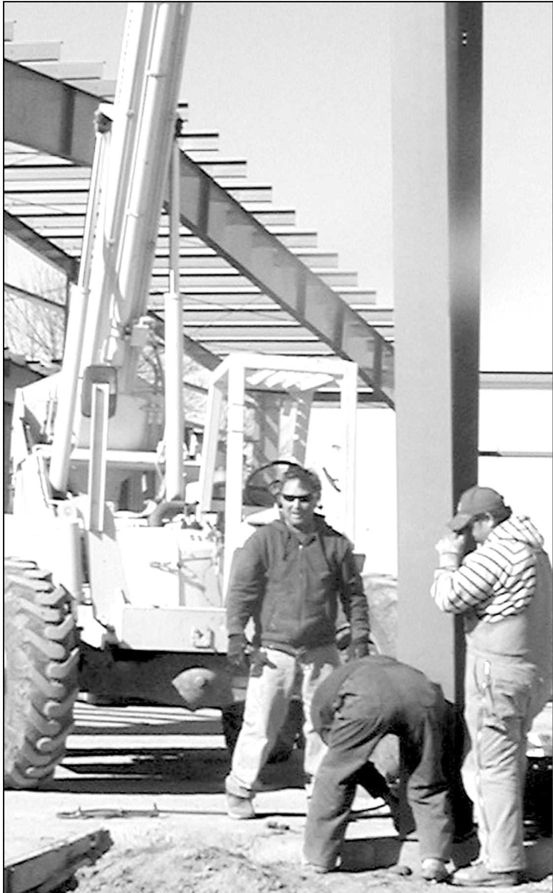
Mike Miller (left), owner of Miller Construction, worked Wednesday with two members of his crew to get a steel corner post in place on the southeast edge of the shop expansion on the Diesel Technology building at the Northwest Kansas Technical College. The addition will add room to work on up to eight trucks or four-wheel-drive tractors and two larger doors to handle the bigger vehicles.
