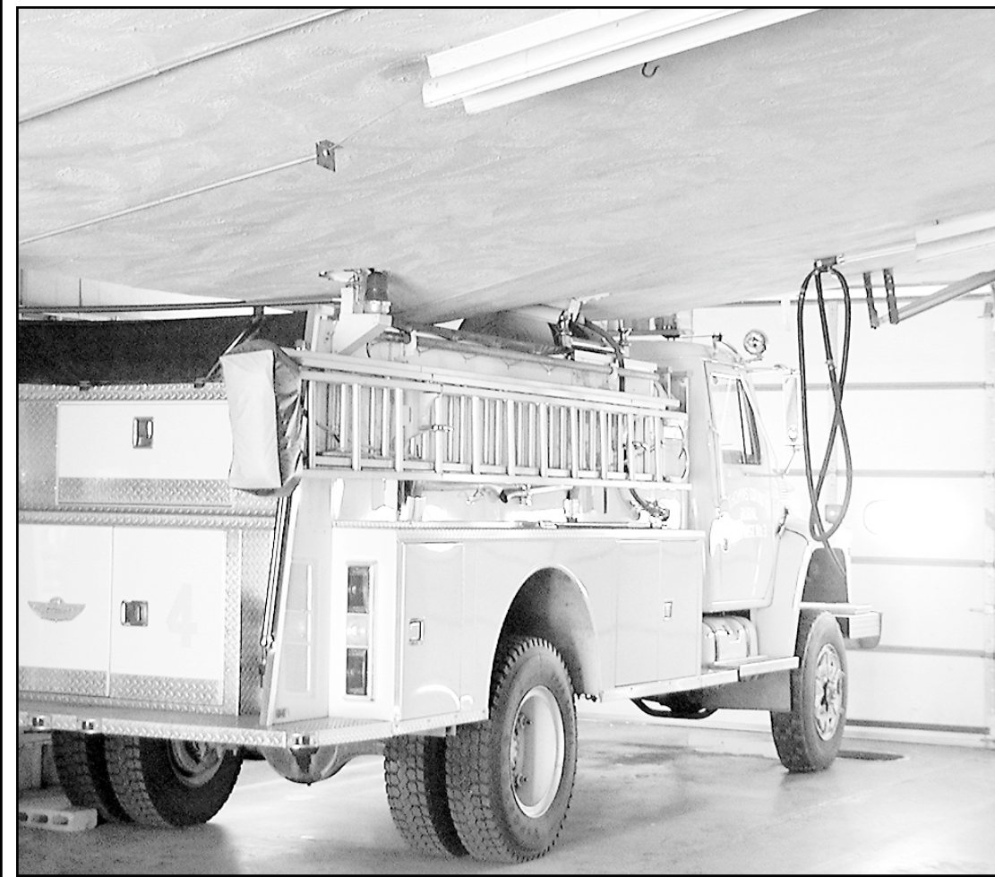
A Colby Fire Department fire truck held up the collapsed roof at the firehouse Sunday after the roof buckled under the weight of snow. Photo by Randy Decker/Colby Free Press
