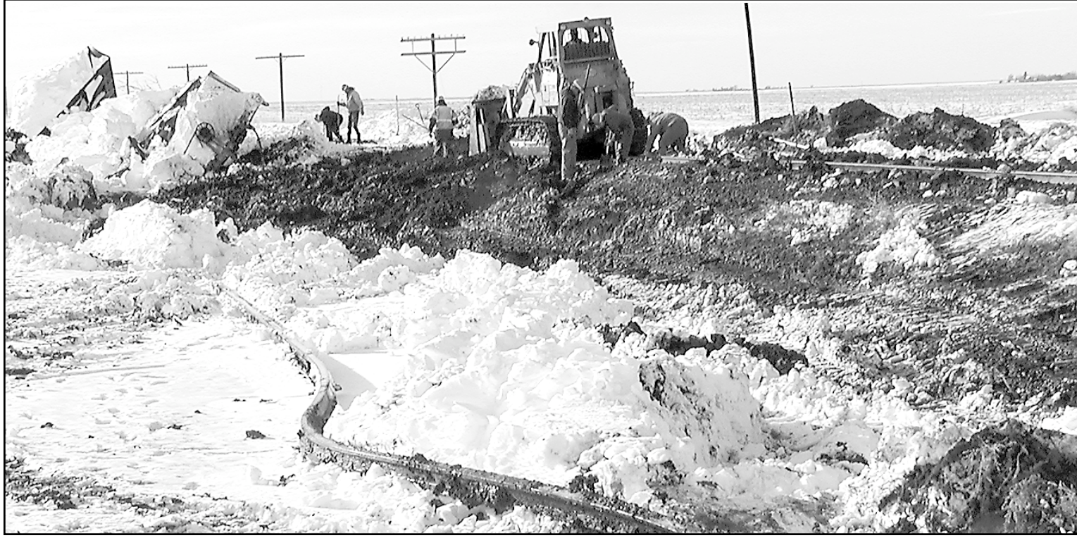
Kyle Railroad track crews worked Wednesday to repair a section west of Kanorado where a snow plow and two engines derailed on Tuesday. The track was repaired by Thursday morning. Photo by Tom Betz/The Goodland Star-News
