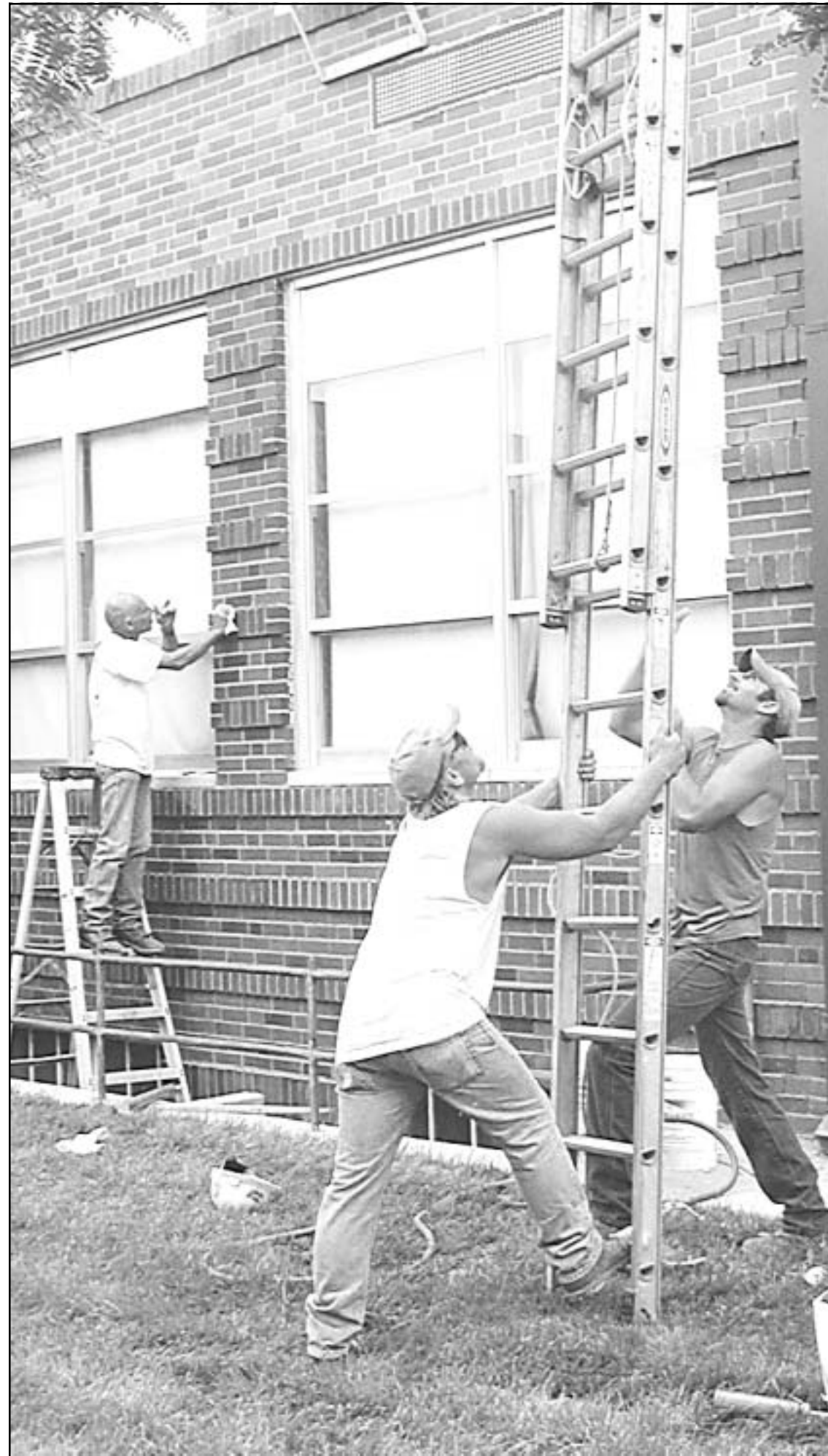
Rodney Lorentz and Ron Durbin Jr. wrestled a 20-foot ladder into place on the front wall of Goodland High School, as Ron Durbin (left) caulked the windows. They are members of crew from Midcontinent Restoration of Fort Scott which has been repairing the bricks at the school, and will be spending six weeks doing the same type of repairs at the Sherman County Courthouse.
