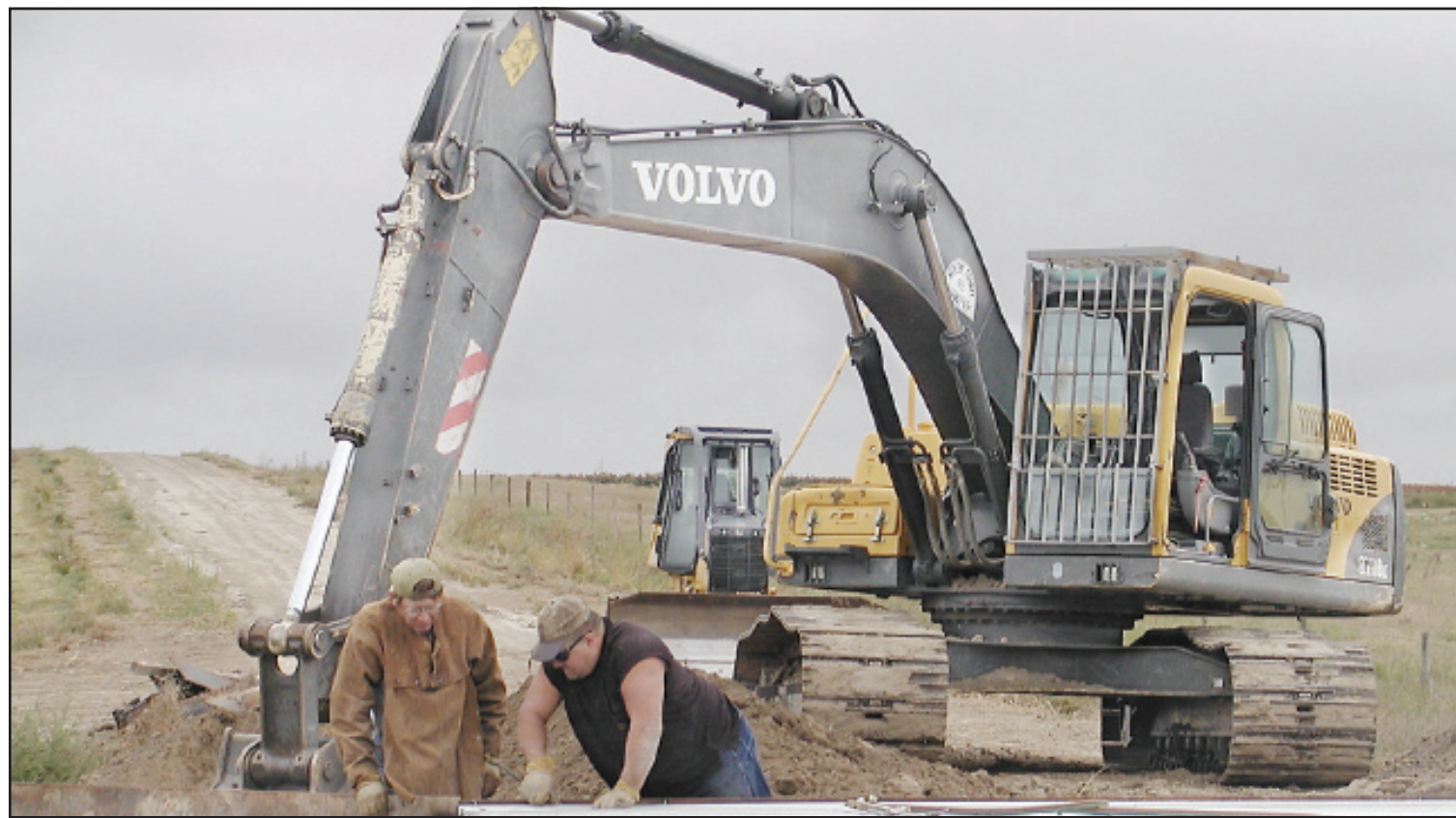
Norton County Bridge Foreman Mark McKenna and a Norton County Bridge crewman installed a new bridge north of Norton this September. The new bridge replaces a county bridge that was in disrepair and replaced on the recommendation of the Federal Emergency Management Agency. – Photo by Carleen Bell/Norton Telegram
