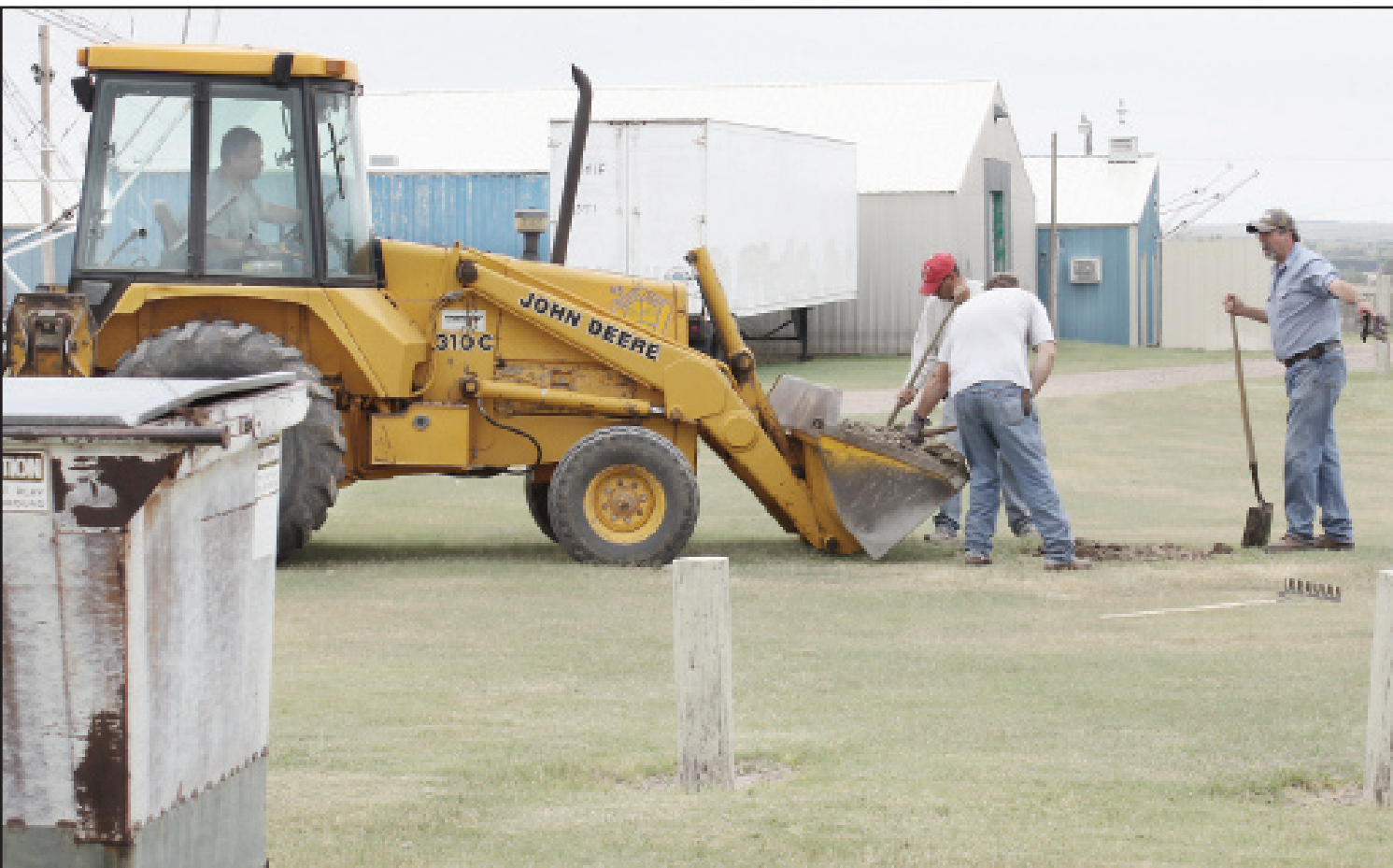
Decatur County Road and Bridge crew members worked at the Decatur County Fairground this summer filling in holes to help get the area ready for the fair in August. – Photo by Kimberly Davis/The Oberlin Herald
