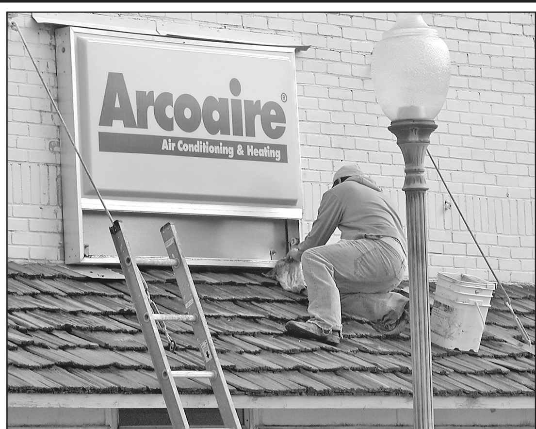
TERRENCE LAMB, Heartland HVAC employee, changes the sign to reflect the new store name.
