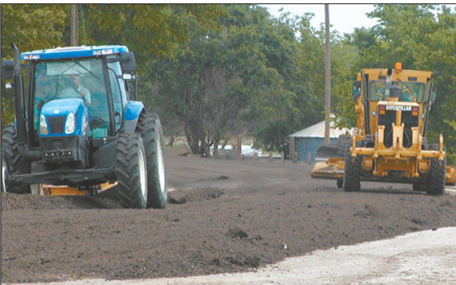
COUNTY CREW spread millings from the K-27 highway project, making the road out to Keller's Pond safer and easier to travel.
