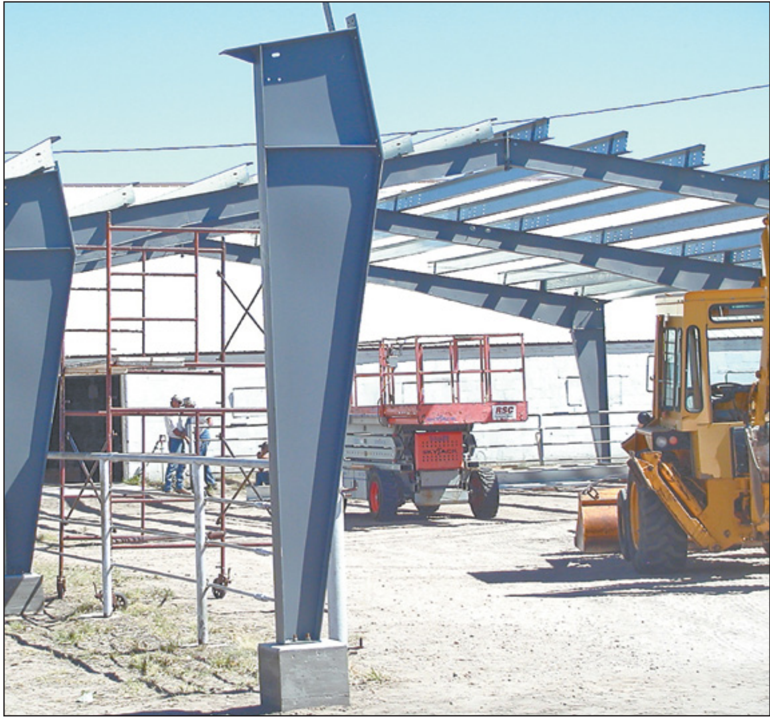
THE NEW ROOF for the livestock arena will be up and ready for the first livestock event at the fair. Ron and Wade Krien, Krien Steel Building, said they would have the building up in time for the fair and they have worked steadily since the building came in on July 9.
