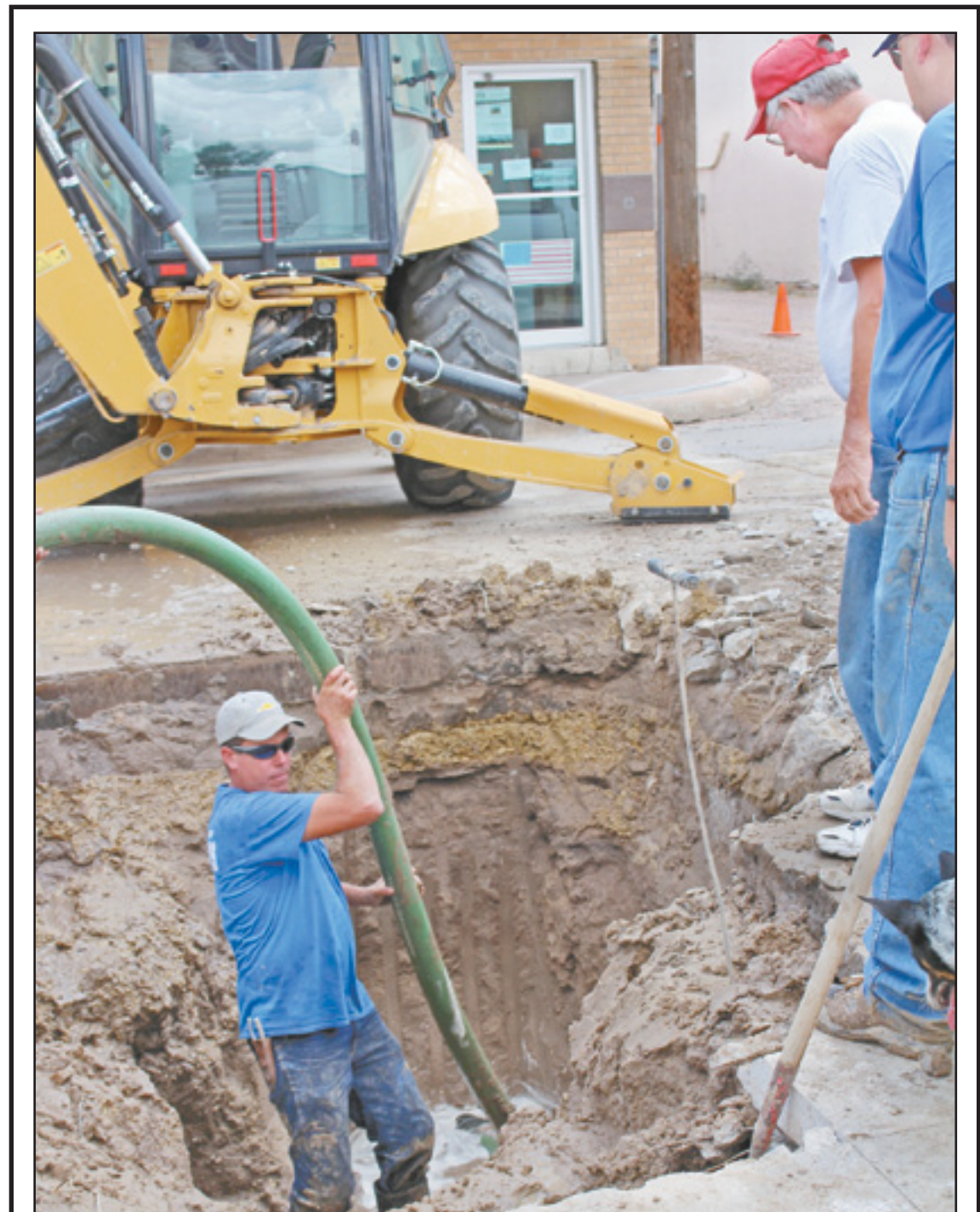
CITY CREW was called to Quincy Street in front of Bier's Hometown Store and Kelly Lampe's shop to fix a broken water main. The city was without water for only about 30 minutes. Troy Meyer is getting the hose to the water, so it could be removed and the main fixed.
