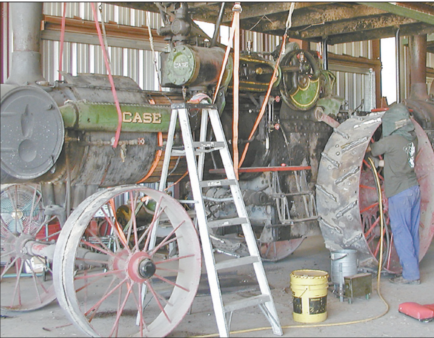
LLOYD STOVER, Pueblo, Colo., is sandblasting spots for the ultrasound to test the boiler thickness before the Tri-State Engine and Thresher Show starts on Thursday.
