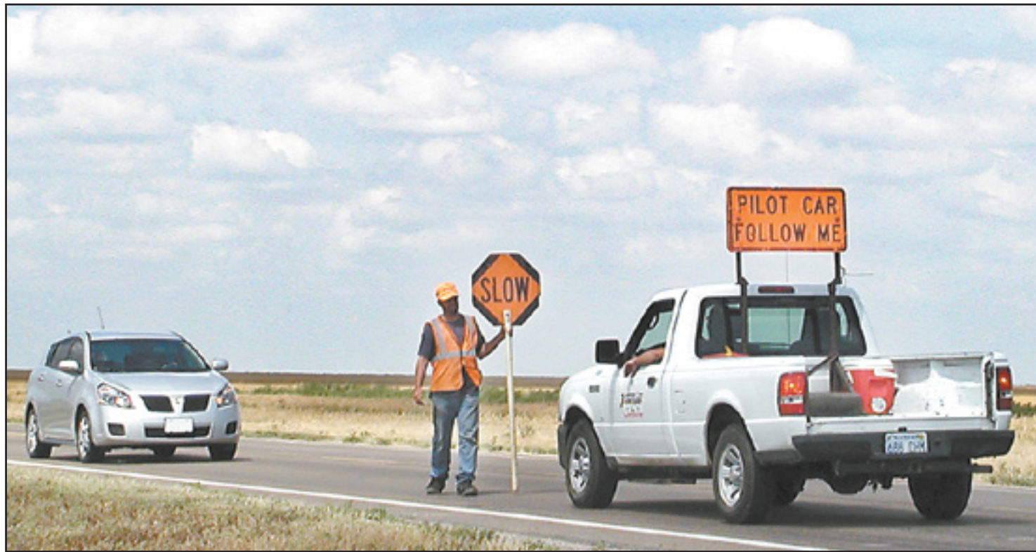
ROAD CONSTRUCTION has begun in Cheyenne County. U.S 36 as well as K-27, both south of Wheeler and north of St. Francis, are being worked on. There should be no more than a 15 minute delay as travelers will need to follow pilot cars. Drivers are urged to drive carefully and give workers "a break!" Herald staff photo by Norma Martinez
