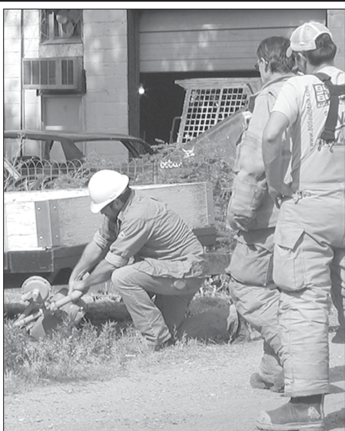
GAS METER hit in the alley. Travis Jensen from Midwest Energy, left, gets the gas shut off. Fire chief George Harper and fireman Clay Zimelman were on hand in case of an emergency.
