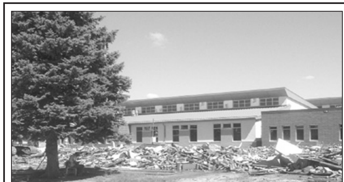
WORK CONTINUES IN IDALIA as the high school wing was demolished, leaving the new school. The new pre-kindergarten through 12th grade school is on schedule to open in August 2013 – in time for the new school year. Herald photo by Nancy Helling
