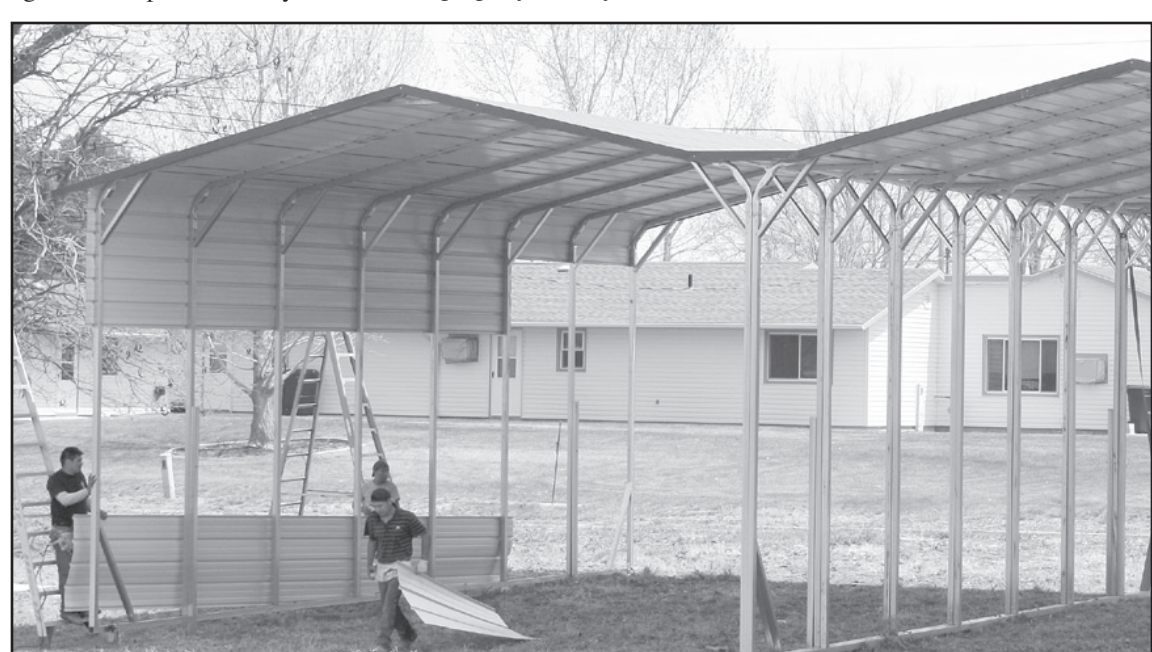
LONESTAR STORAGE recreational vehicle storage is already up and more storage is yet to come. Check the progress on College Street.
