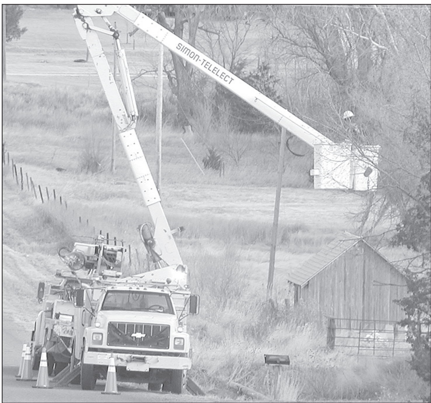
PRAIRIE LAND crew put in some new lines on the old Wheeler Road last week.
