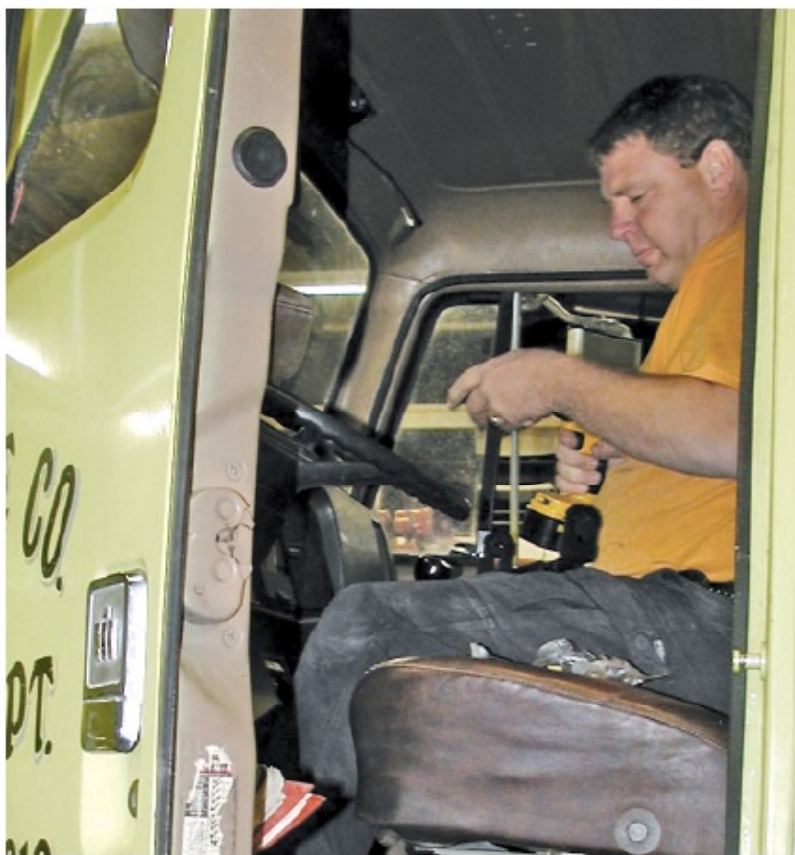
INSTALLING 800 MEGAHERTZ equipment in one of the county fire trucks was Rick Elliott with Prairie States Communications.
