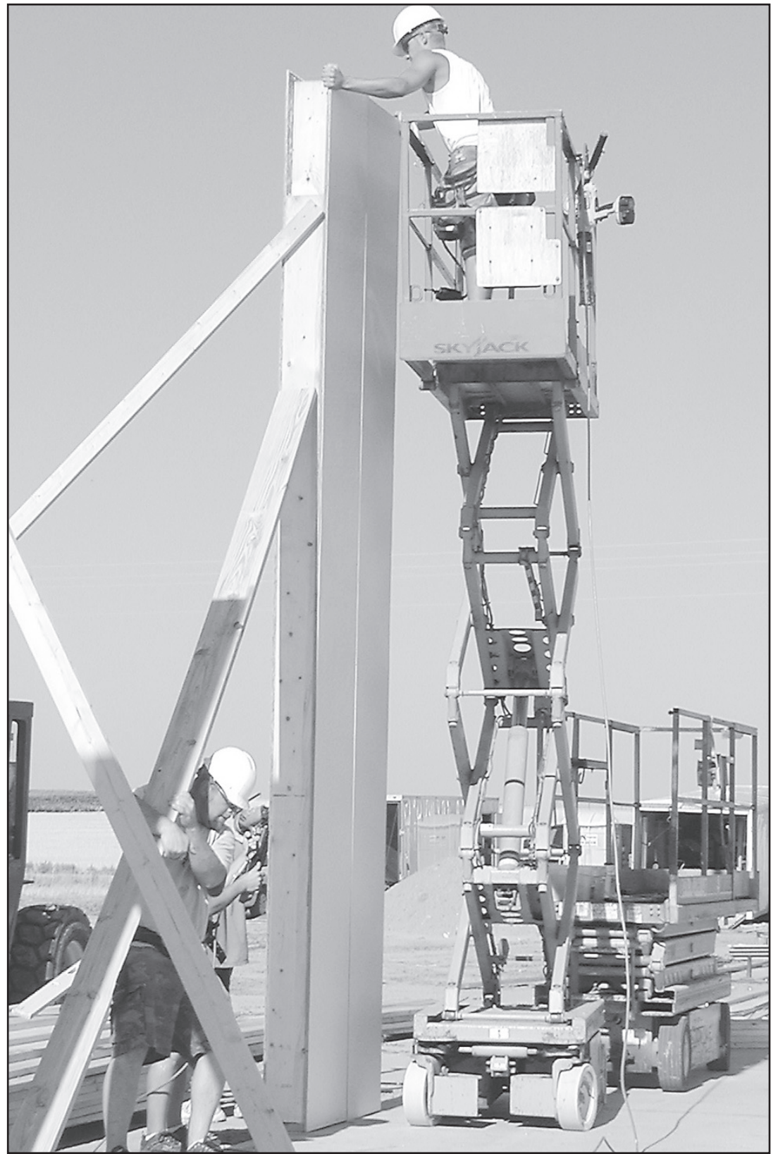
EAST OF ST. FRANCIS, the new PrairieLand building is quickly going up. The business is moving from Bird City to rural St. Francis.
