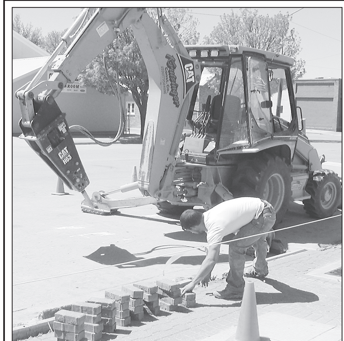
WORK ON NEW CURB and gutter has begun on St. Francis' Main Street. There will be several blocks under construction. The first block is the 200 block of West Washington.
