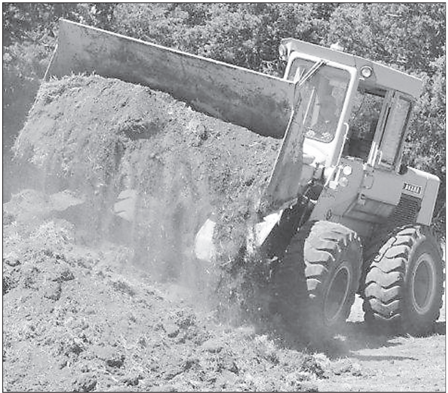
GROUNDWORK BEGAN for the new restaurant and bar in Idalia. The money to build the restaurant was raised by donations and shares. The facility is to be opened by Aug. 1. Herald photo by Chuck Wright
