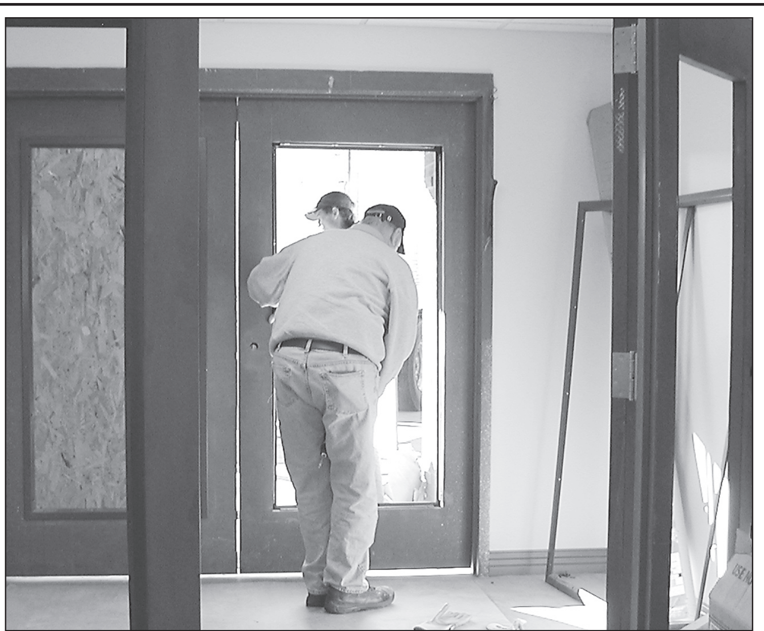
A PROTECTIVE ENTRY way has been added at the Good Samaritan Village. The remodeling is coming along on schedule with the expected finish date of Feb. 1.
