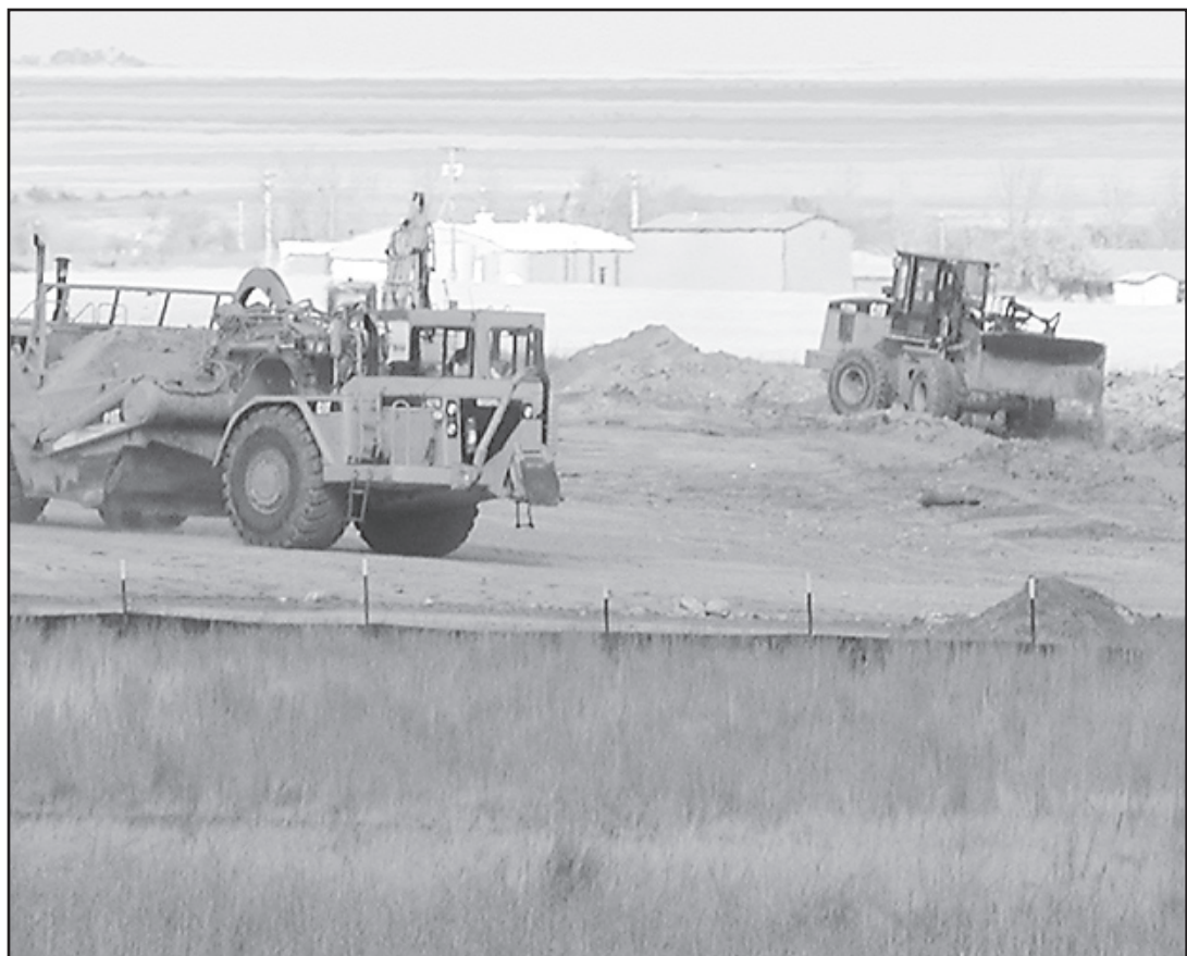
DIRT WORK IS going on at the Cheyenne County Airport for the expanded runway project. Herald staff photo by Tim Burr
