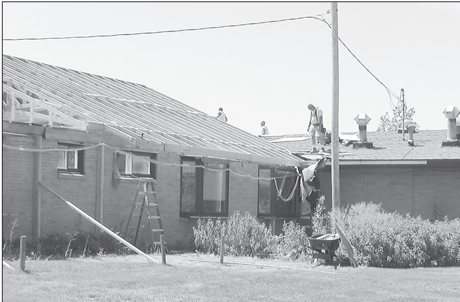
WORK PROGRESSES at the Good Samaritan Village. The underground plumbing has been reconfigured which took some time. Now the roof trusses on the west side are up and the roof is being covered. Getting the new building
