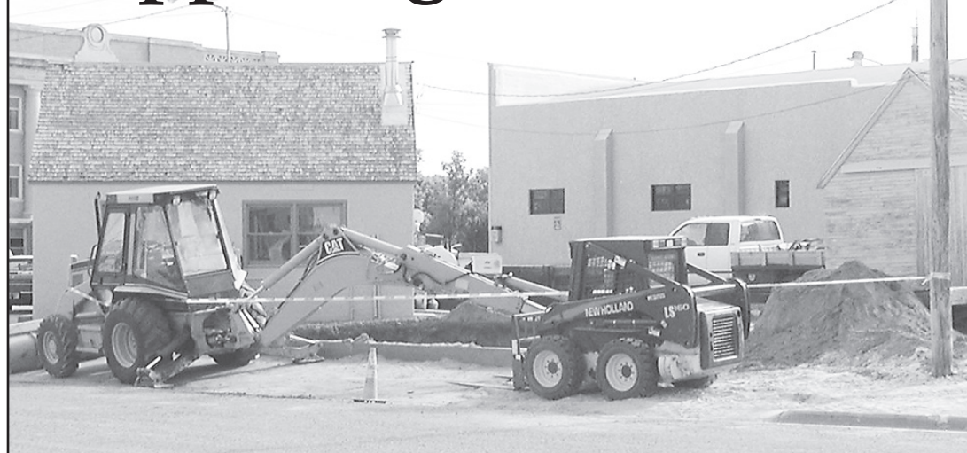
GAS TANKS are being dug up at the Jenik Oil Station. It was announced last week they would no longer be selling fuel.
