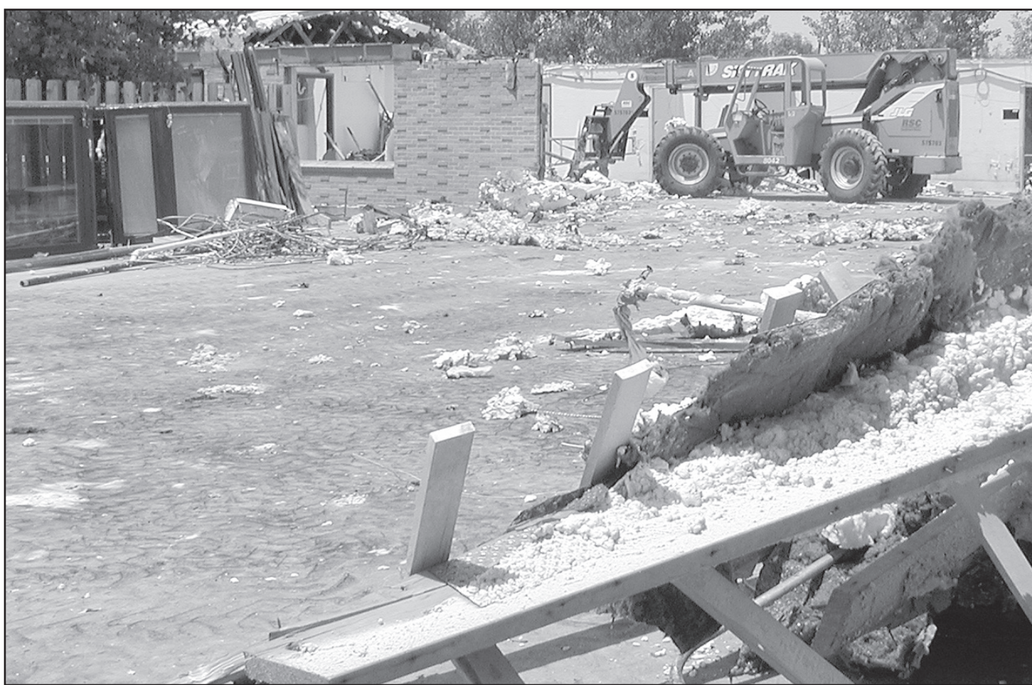
DEMOLITION CONTINUES at the Good Samaritan Village. Jeff Paulsen, Village administrator, said the crew is about half done with the demolition of the middle section which was destroyed in the Oct. 19 fire.
