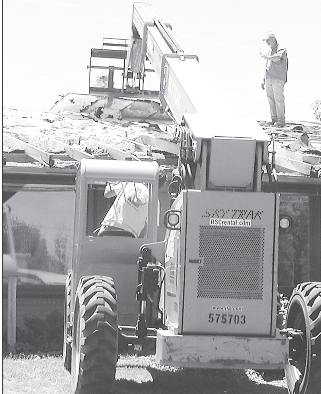
AFTER MONTHS OF WAITING, the roof on the Good Samaritan Village's burned section came off. A wall will be demolished and the middle section where there was severe fire damage will be made into three private rooms, three offices and a corridor. See Page 3 of this issue for the story and plans.
