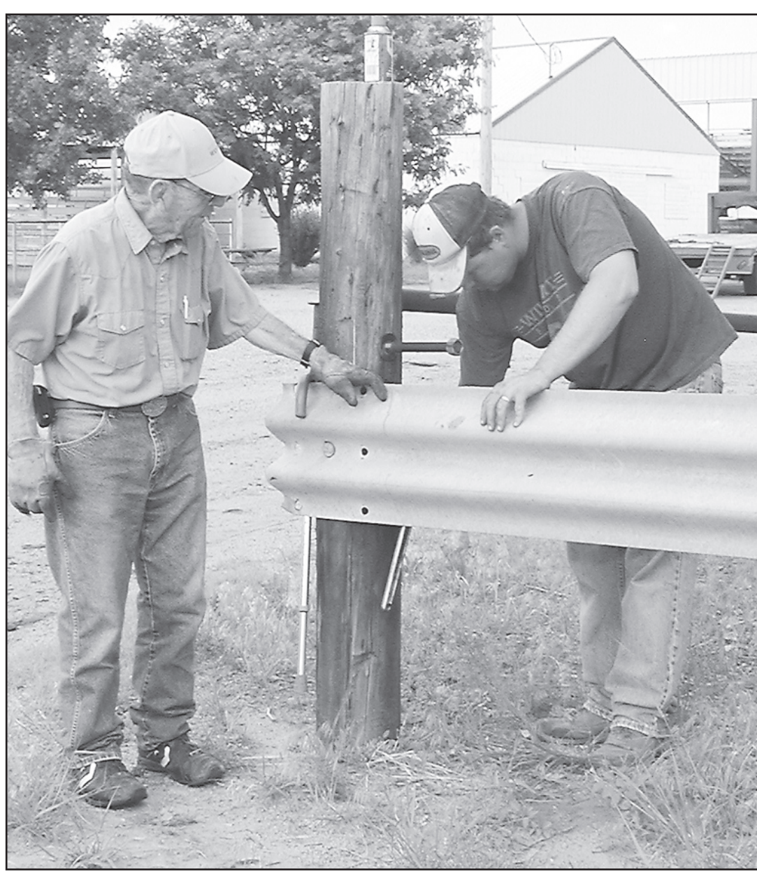
FAIR BOARD MEMBERS were working at the fairgrounds Thursday night. They will be cleaning up, mowing and making last minute repairs before the county fair begins on Aug. 3. Working on a gate are John Finley, left, and Drew Flemming.
