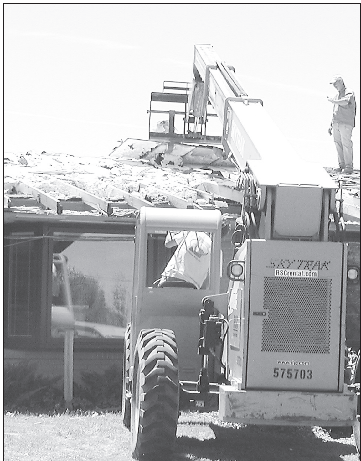
AFTER MONTHS OF WAITING, the roof on the Good Samaritan Village's burned section came off. A wall will be demolished and the middle section where there was severe fire damage will be made into three private rooms, three offices and a corridor.
