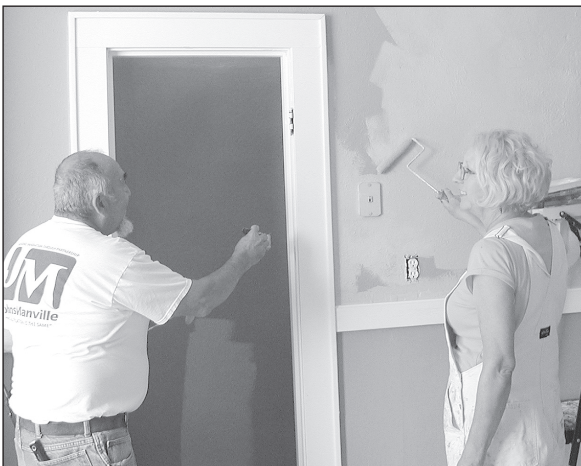
VOLUNTEERING— Willy Martinez and Roseanna Underwood, Century II board member, paints the office in the old Security Bank building.
