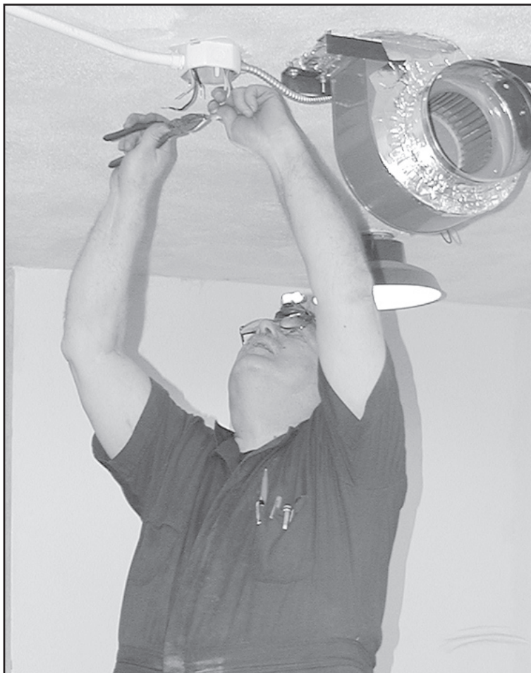
WORKING ON ELECTRICAL boxes was necessary before Dennis Murphy, Claco employee, could start installing the digital equipment. Herald staff photo by Karen Krien
