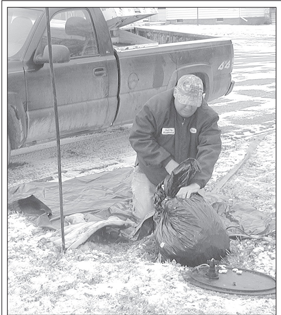
THE FIRST WATER BREAK of the year has happened. Brad Schneider was out on Fourth Street Saturday checking out a leak from a water meter that was not insulated good enough. He said they had 16 breaks last year, and with spring coming, pipes are going to start breaking once again. Mr. Schneider is doing the best he can to keep everyone with water. He is to be commended for the good job he has done in keeping the streets repaired from the breaks, and has done a super great job of keeping them clear during the snow storms.
