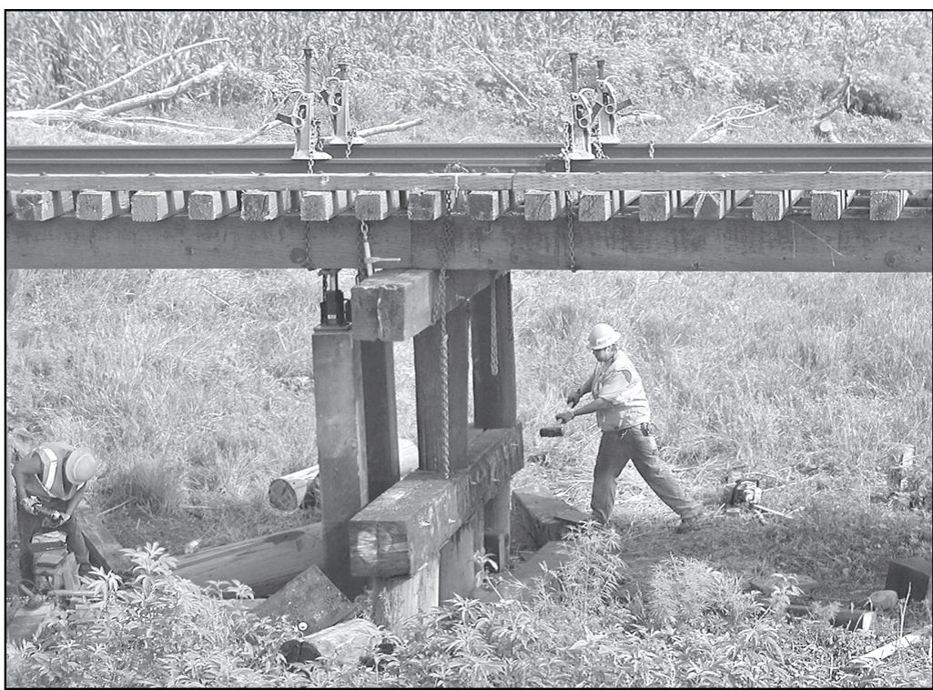
Among the casualties of a string of tornadoes that struck the area on June 20 was this wooden railroad bridge northwest of Almena. The bridge was damaged by the tornadoes and Tyson Construction of Norfolk, Neb. spent Friday morning repairing the damage. Among other things, the construction included replacing broken weight-bearing beams under the main span of the bridge.
