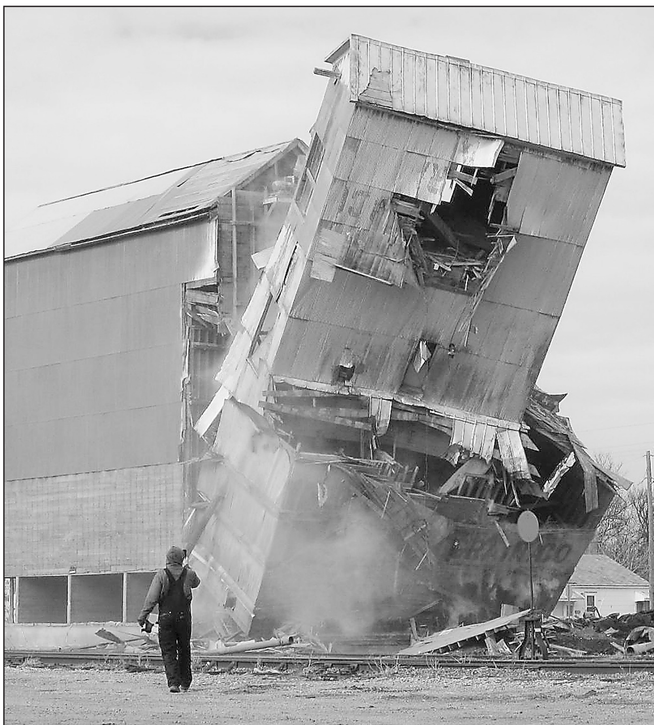
A worker from Forest River Colony and Salvage, Fordville, N.D., watched as the old Brady elevator was demolished on Wednesday afternoon. The elevator had been leaning, and had been a source of concern for people in that area of the community. The elevator was located just across the street south of Walter Motor Co., which is located at 124 S. 2nd.
