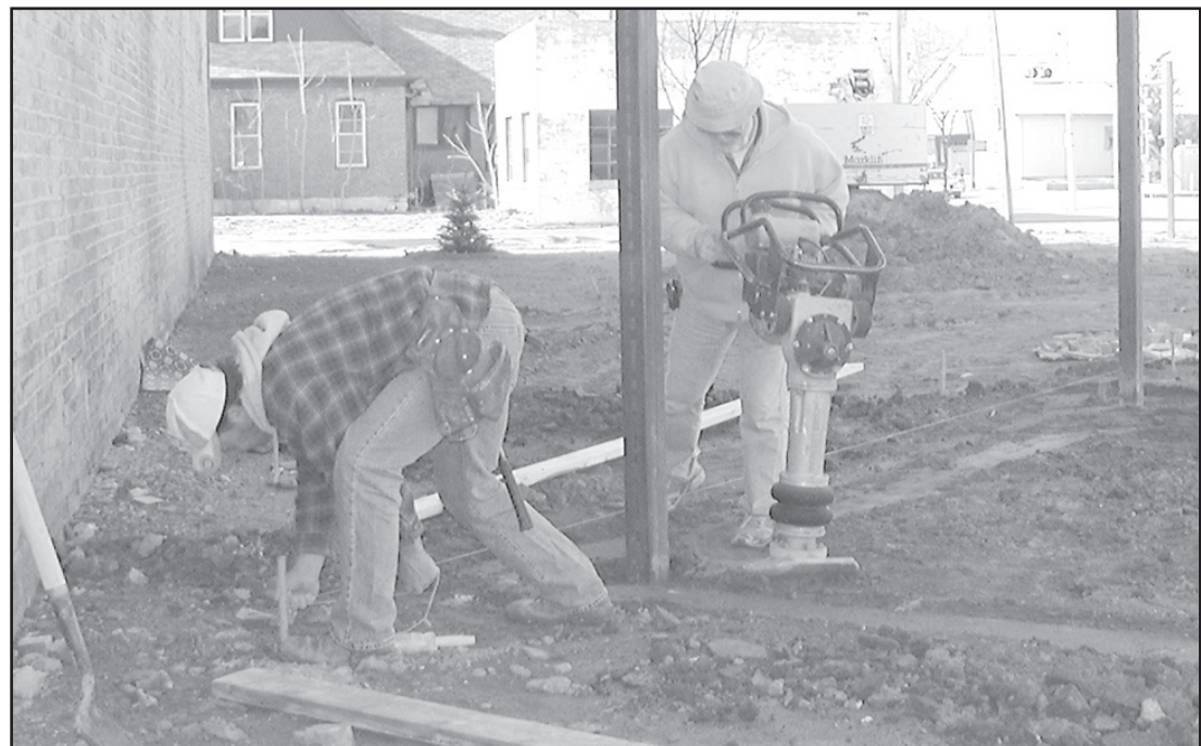
Kirk Griffith and George Jones of Custom Flatwork laid out the forms and tamped the soil in preparation for the concrete decks that were poured this week at the new downtown park. Other plans include pergolas over the decks, a fountain in front of the rocks and a brick sidewalk.
