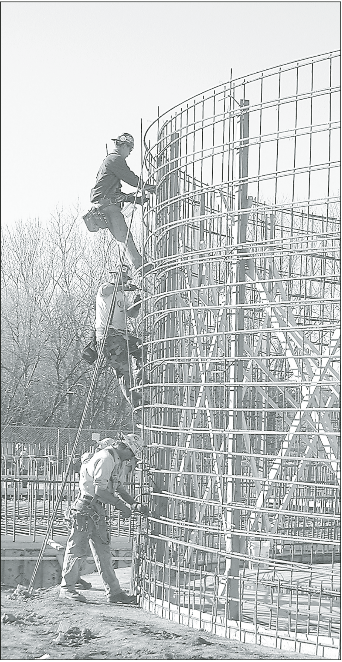
Steel workers subcontracted through BRB Contractors tied steel in place around the east counter-current aeration tank. The tank is one of two that will make up part of the new sewer plant for Norton. The $3.6 million project has to be completed by next August.
