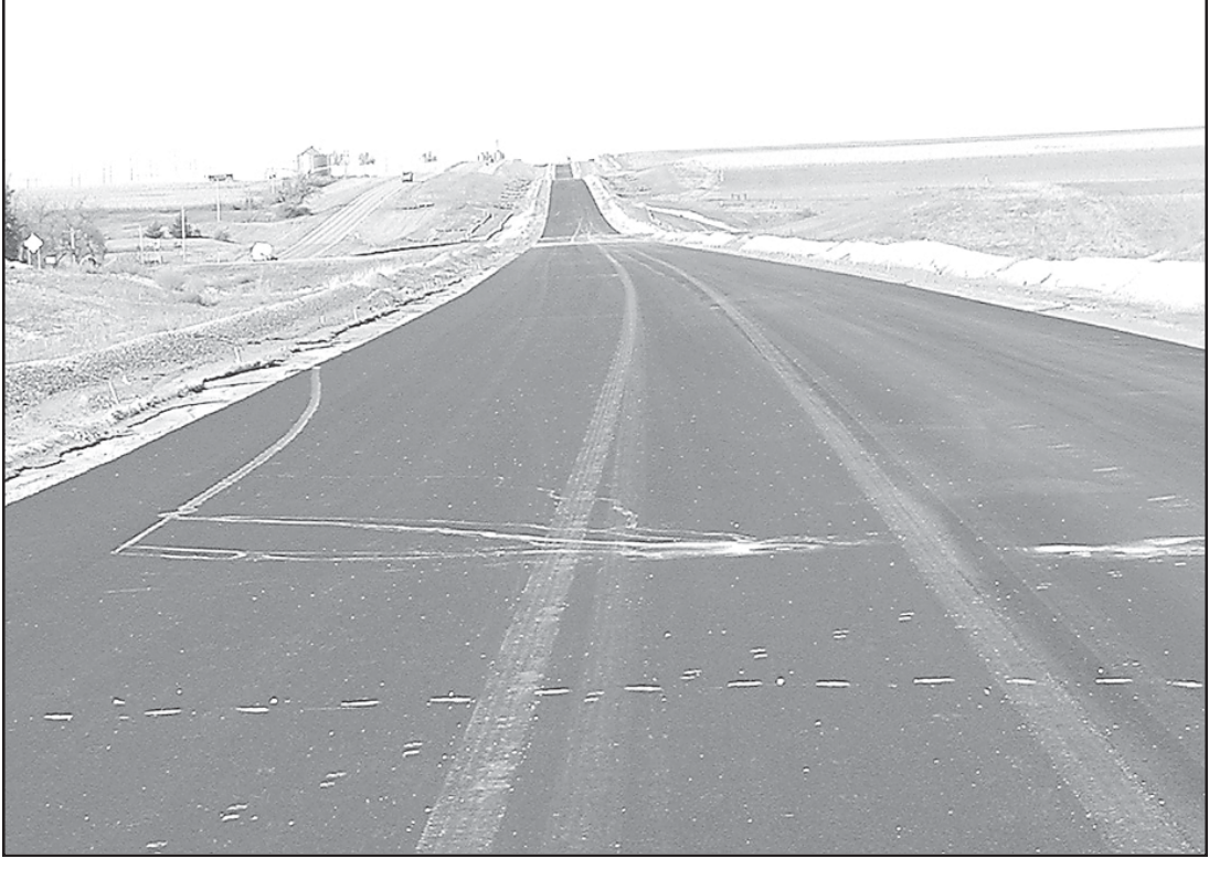
Highway work continued on U.S. 36 six miles west of Norton. This stretch of blacktop was just recently completed. — Telegram photo by Carolyn Plotts
