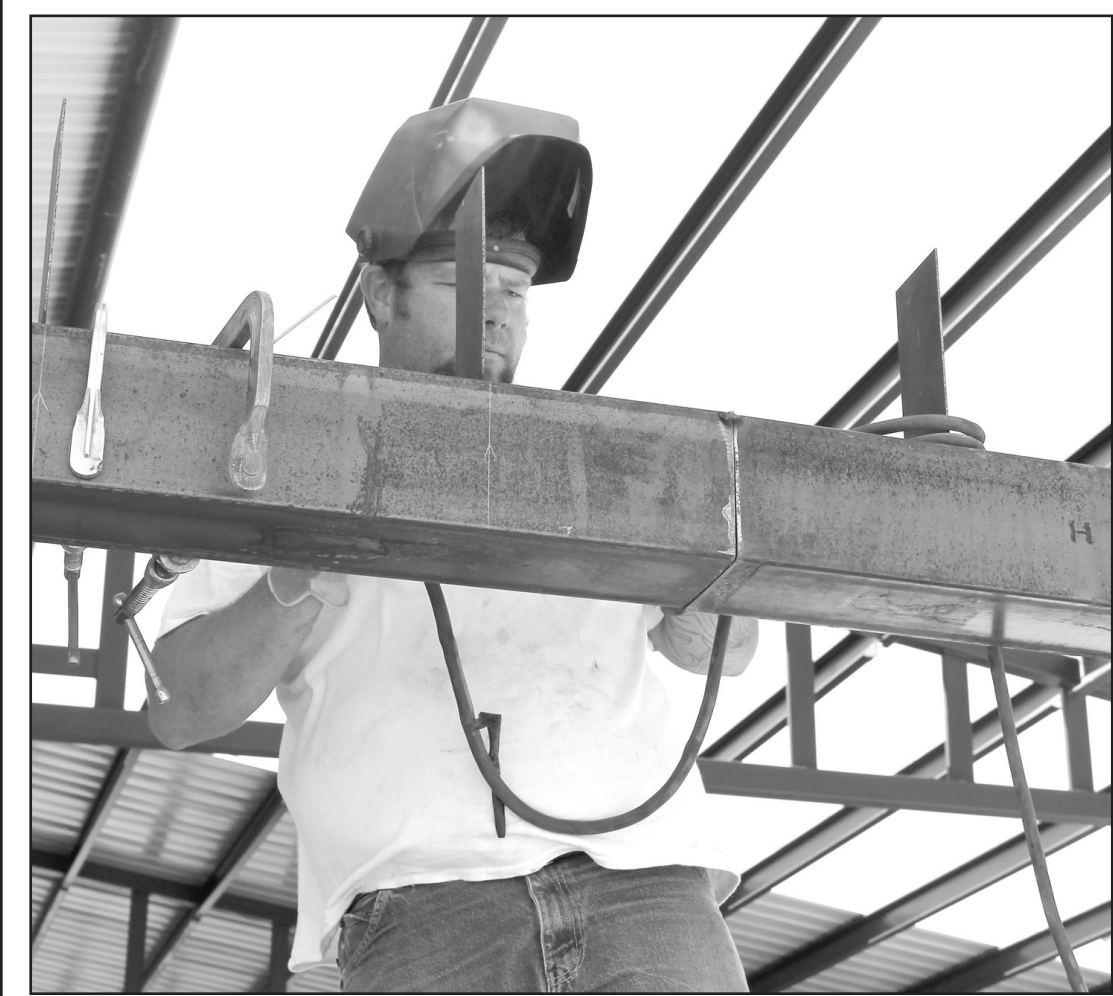
ANDY LIMING and his crew from Wray, Colo., are diligently working on the new Wright Building to have it ready for the Thresher Show. Andy was welding the left framework, and his crew members were working in the heat on the roofing. Mr. Liming said the building should be done in time, the only hangup might be with the electricity.
