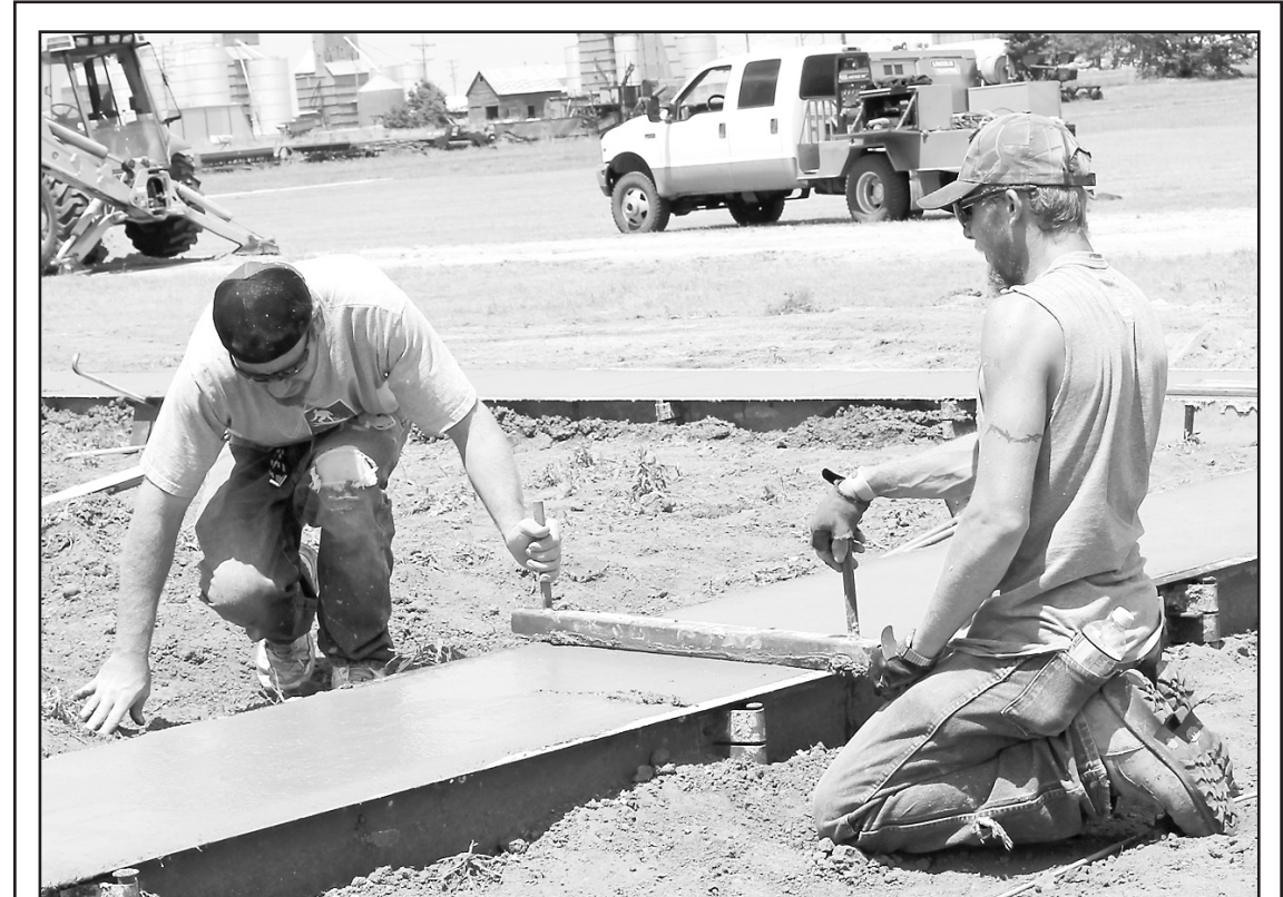
ANDY LIMING with Liming Construction and his crew from Wray, Colo., were at the Thresher grounds, pouring and finishing off the cement foundation for the new Wright Building last Thursday.
