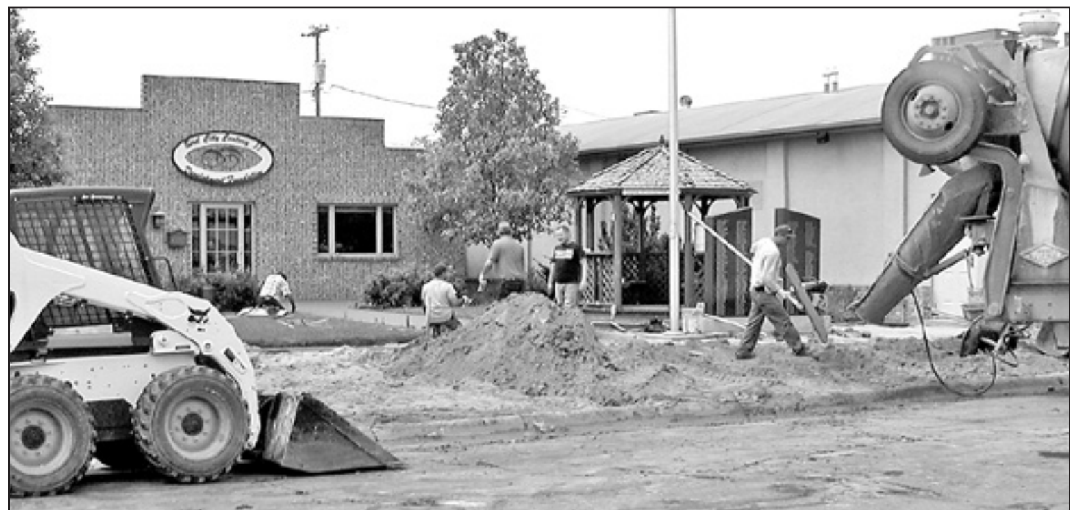
CEMENT IS BEING POURED and many other projects are going on in the city of Bird City.
