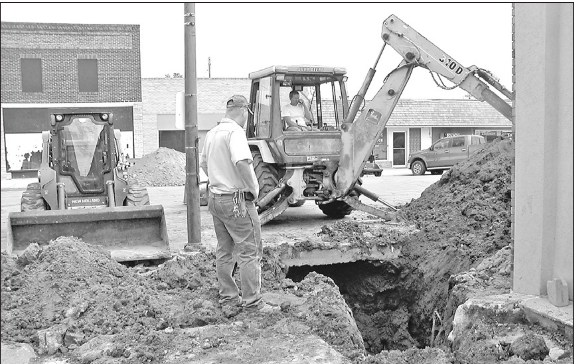
LAST WEEK CITY WORKER Robert Sharp and Roy Shrader were digging in front of the Post Office and Legion Hall to repair a pipe broken by PBC Construction who was tearing out and replacing curbing and sidewalks.
