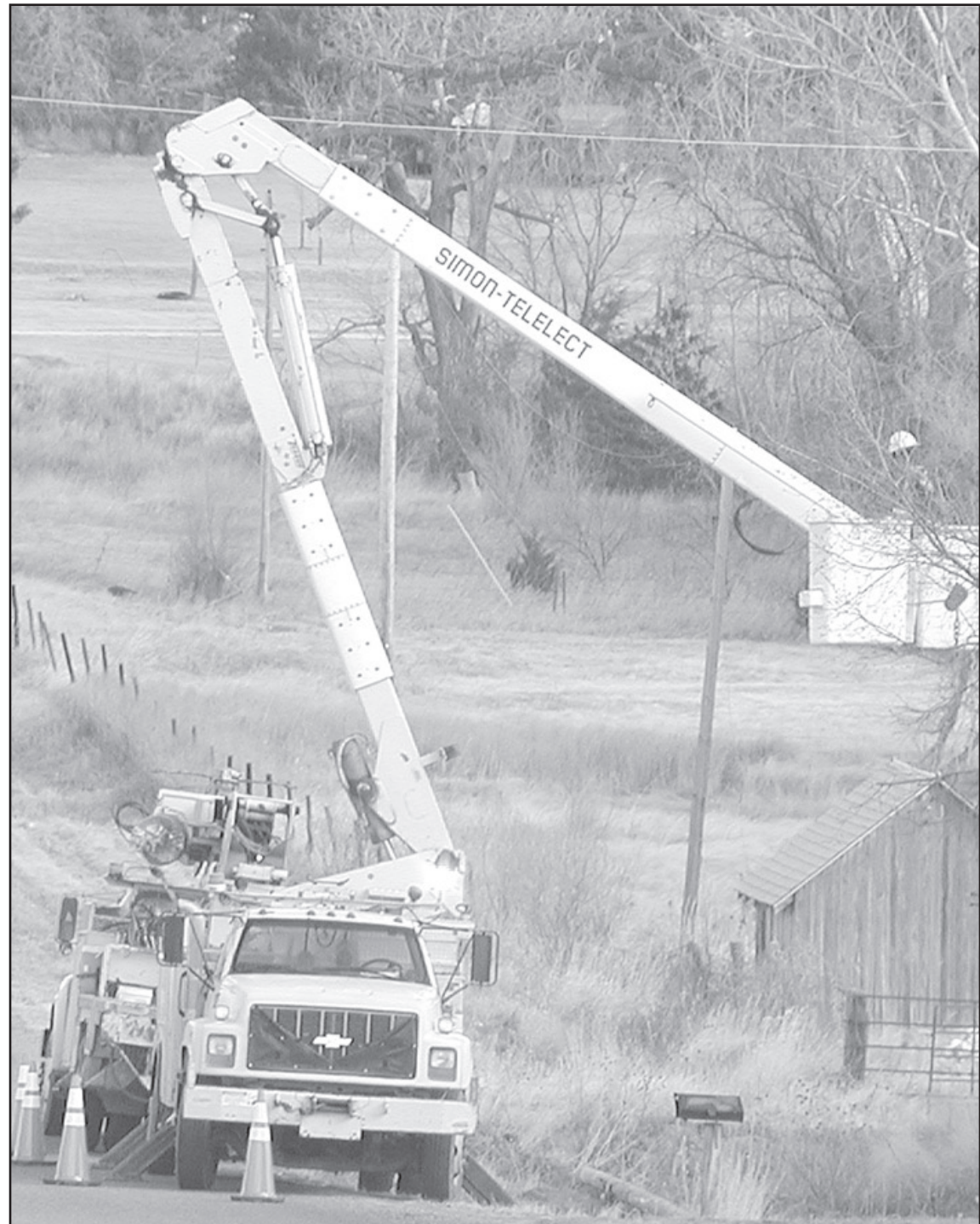
PRAIRIE LAND works quickly to replace power lines before more high winds arrive.
