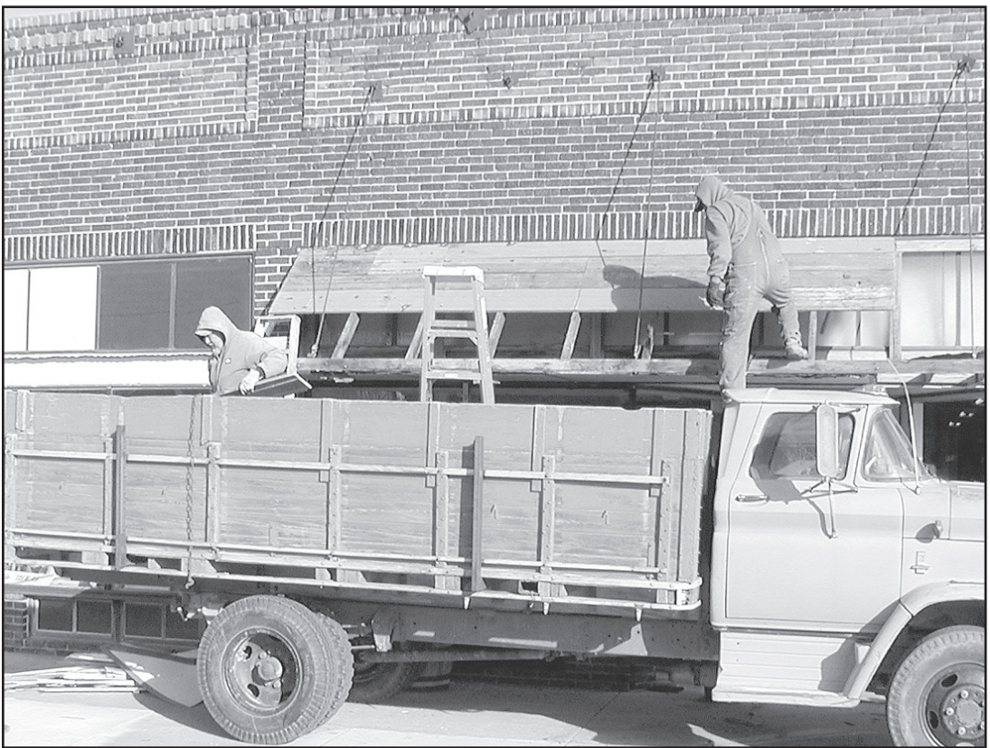
THE SENIOR CENTER is ready for the new awning to be installed after Larry Shults and Willy Martinez removed the old one. Times staff photo by Norma Martinez
