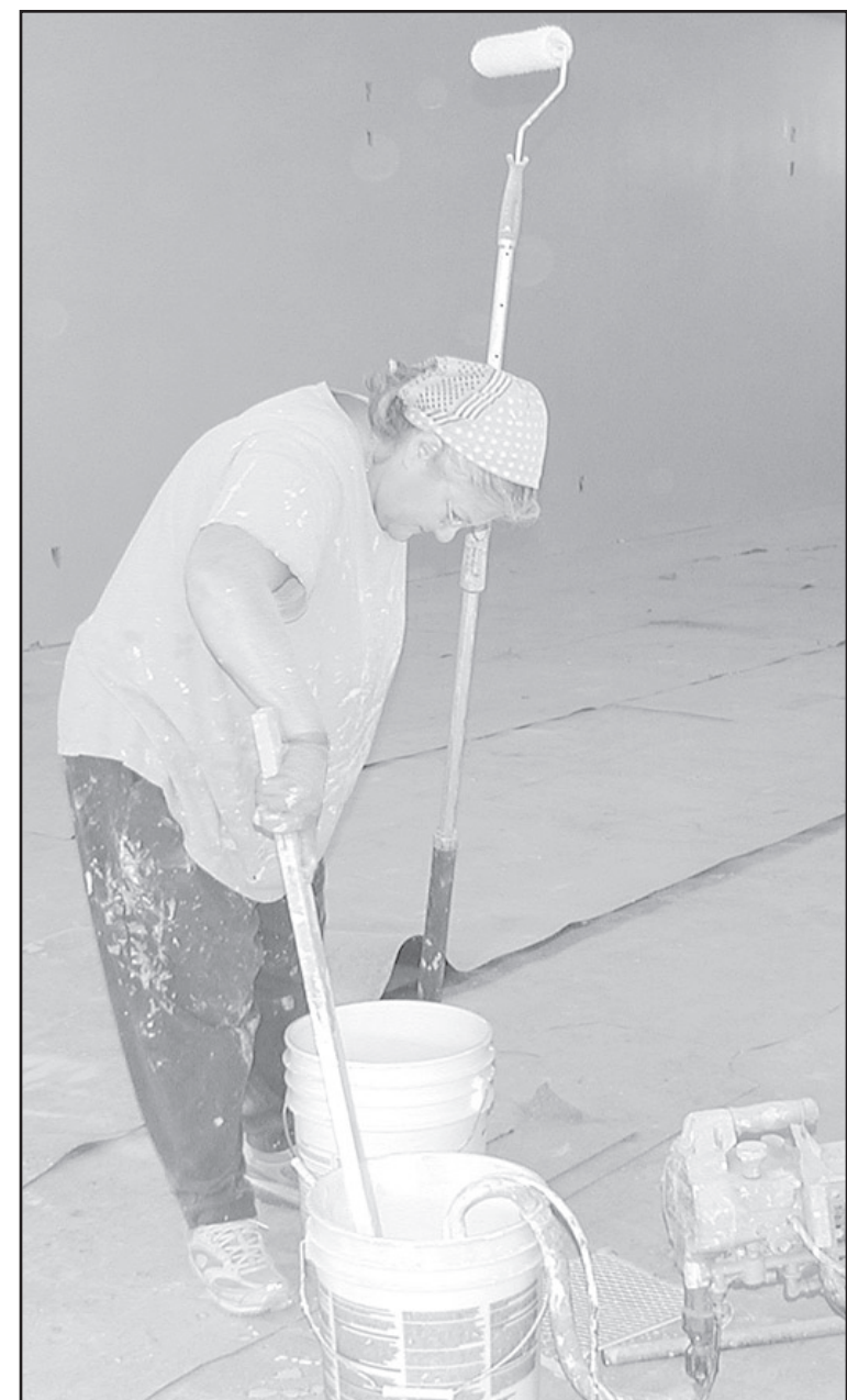
JAN BUSSE is turning white while rolling paint on the walls and ceilings to the Wellness Center.
