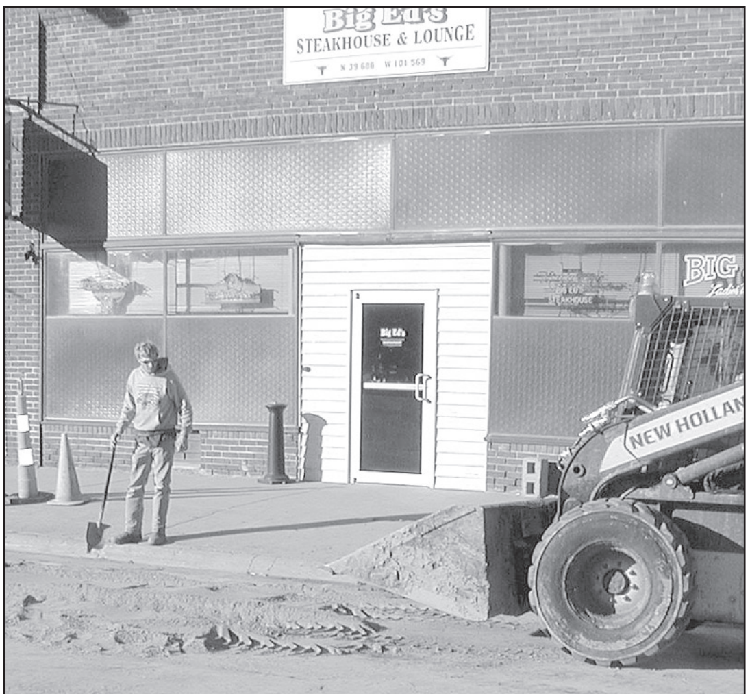
BRENT WHITTINGTON Bird City part-time worker, and Brad Schneider , supervisor, cover up the hole from the second waterline break in 2013.
