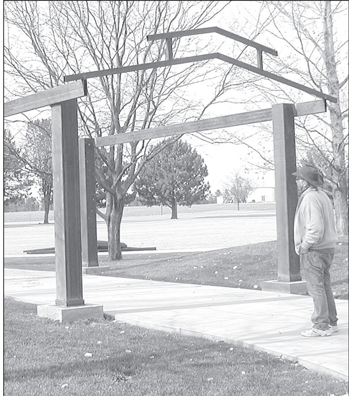
STAN DORSCH checks out Rod Young's welding work on the pergola being installed at the park.
