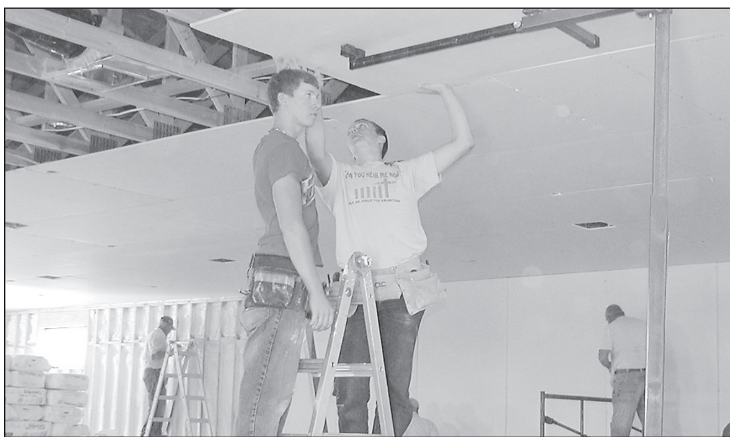
GRANT SHRADER and Shaun Pochop from Industrial Arts are installing the ceiling tile in the Wellness Center. Times staff photo by Norma Martinez
