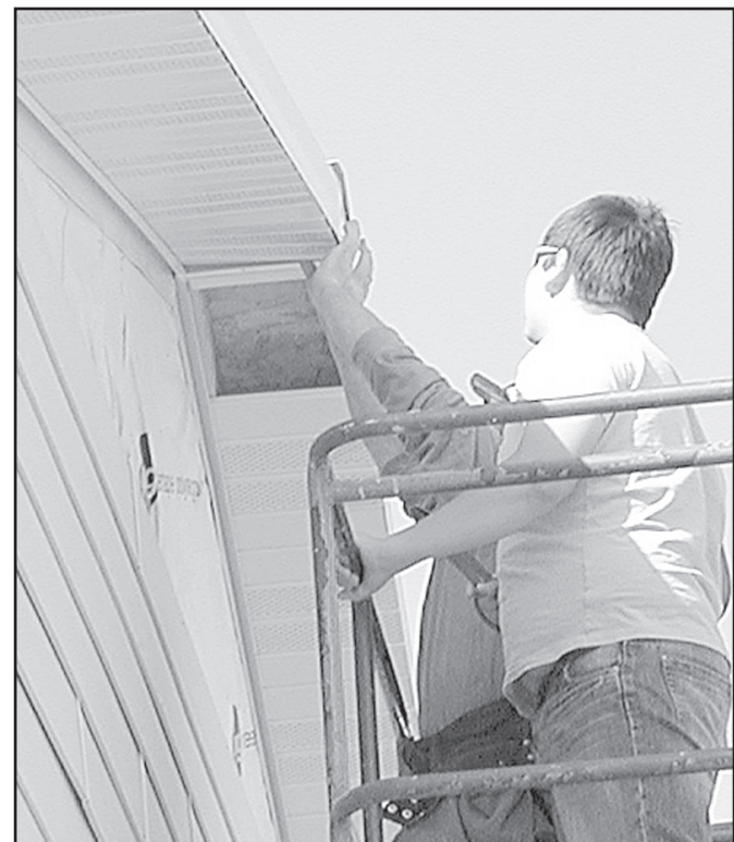
BRIAN PERKINS and Eric Estrada nailing siding on the north top of the Wellness Center.
