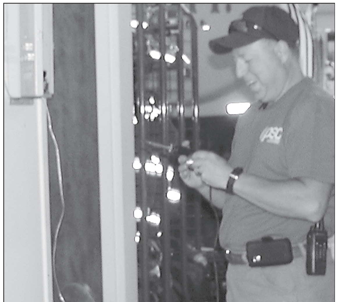
BILL WHITLOW is hooking up the wiring to the emergency siren system, so it will be compliant to the Federal Communications Commission for Narrow Banding.
