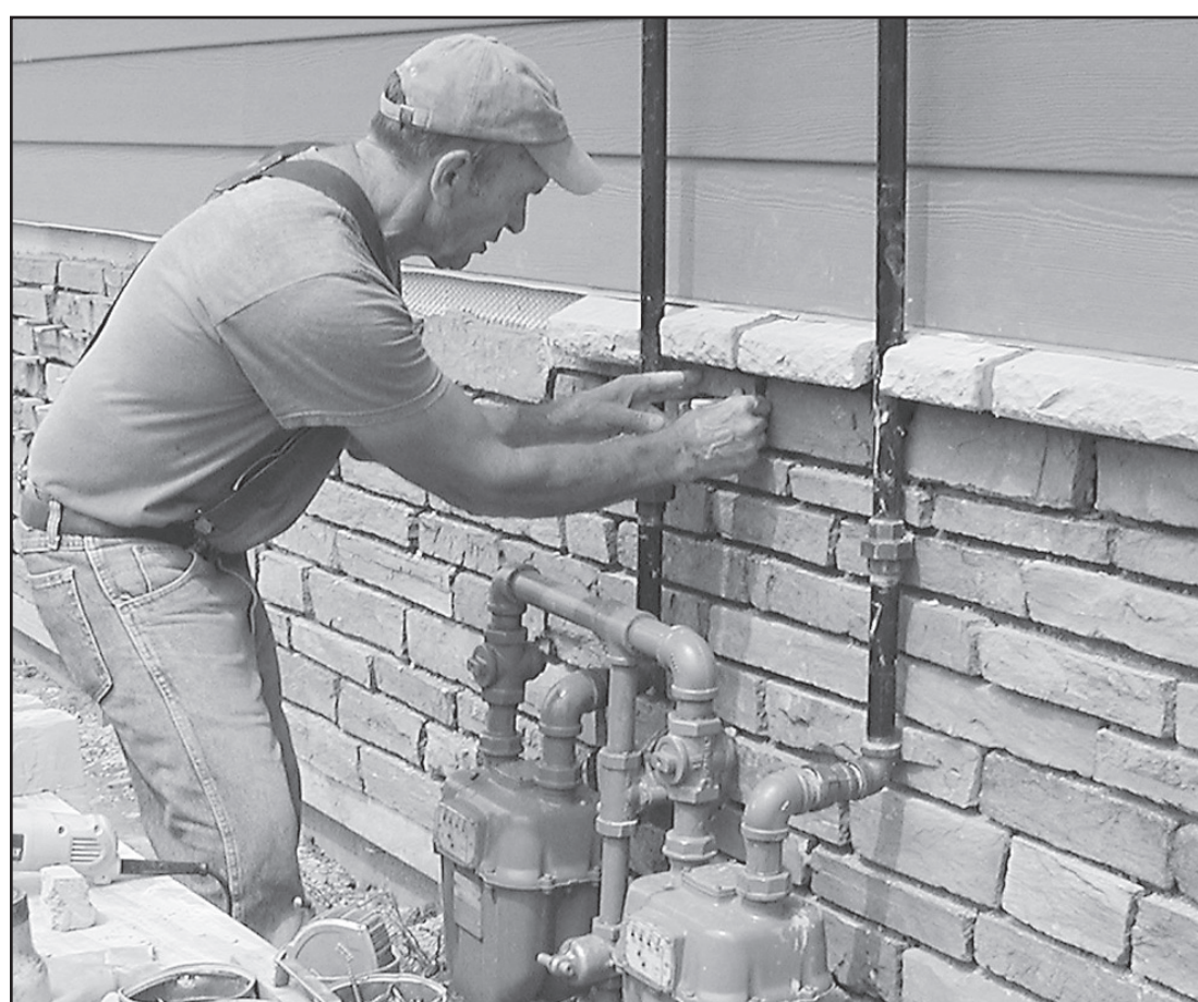
JOE CHECK with Check Construction from Goodland is putting the artificial brick on the first unit of the Senior Housing Unit. Construction workers are hard at work with plans of having it completed by October 1, for the first resident.
