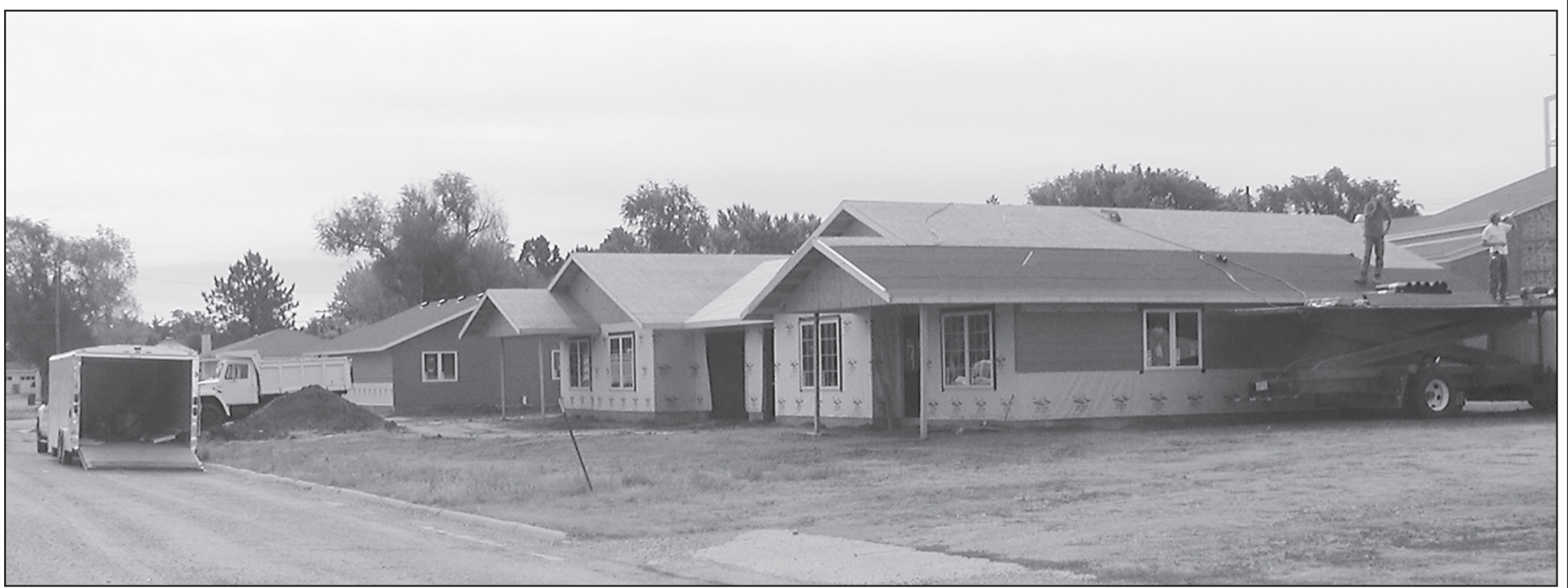
CONSTRUCTION IS well underway on the double unit apartments at the Bird City Senior Living complex.
