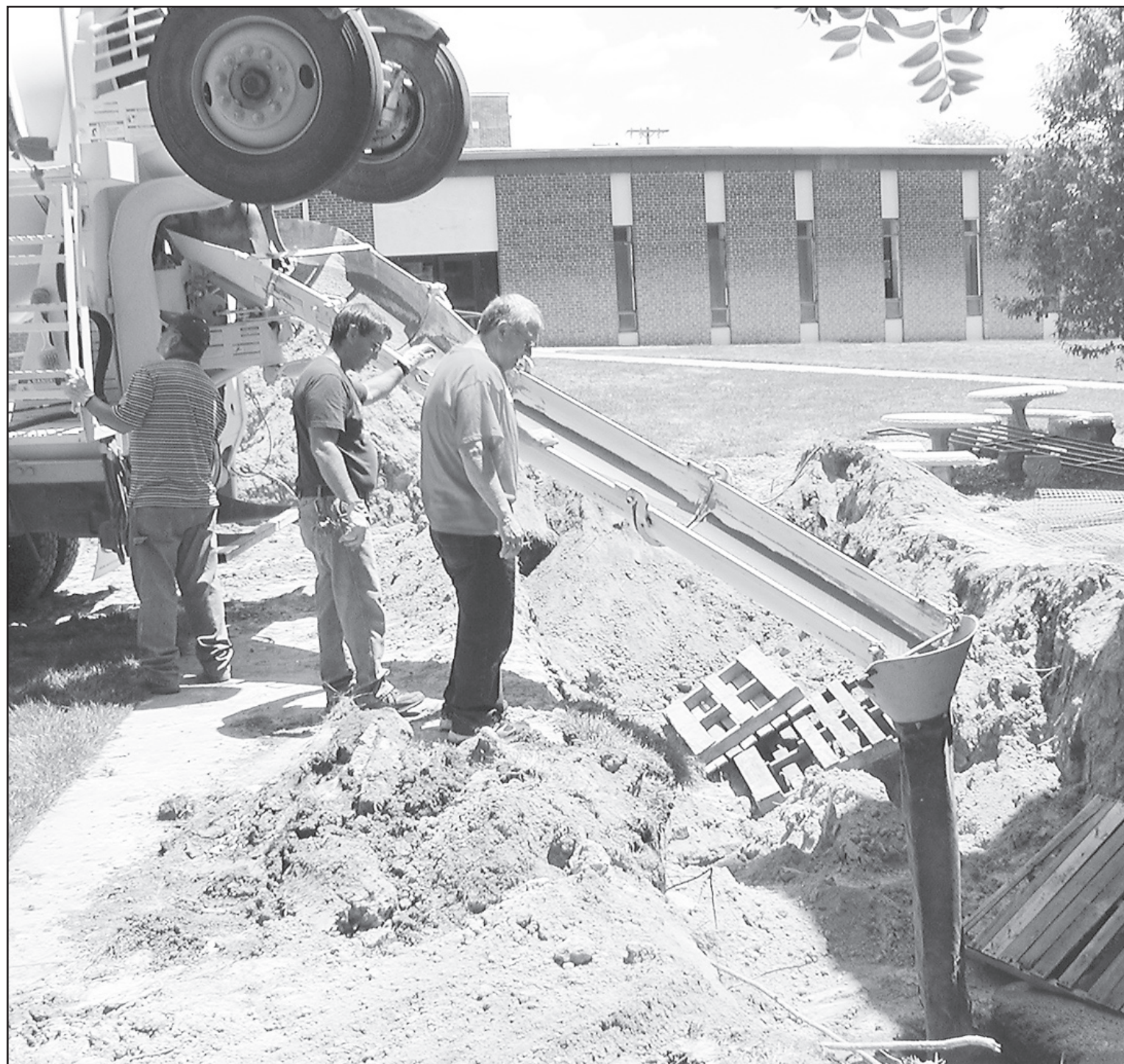
BRUCE Bolin and Randy Miller are pouring cement to fill up sink holes which appeared next to the Cheylin High School.
