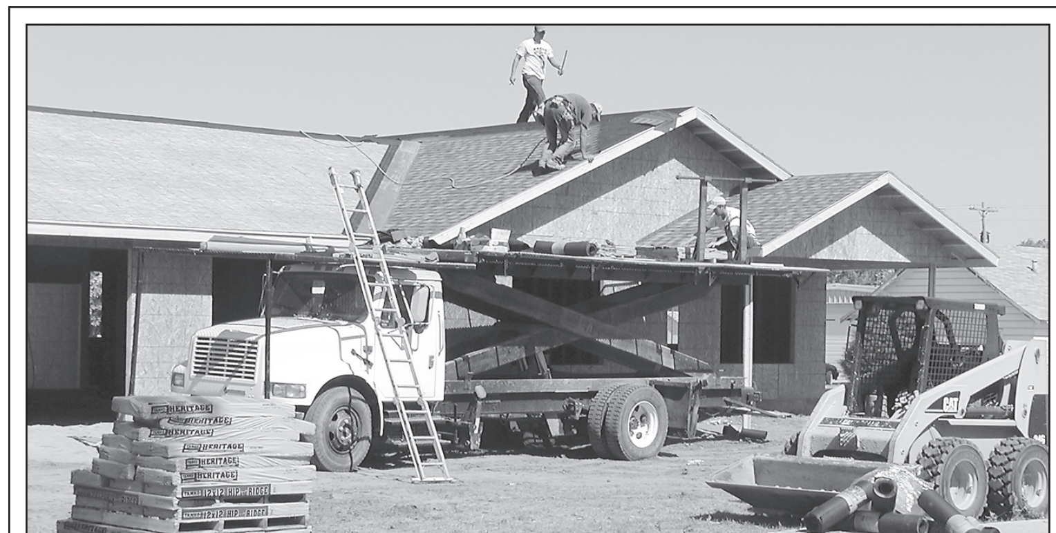
WORK has started on the new senior independent living apartments in Bird City.
